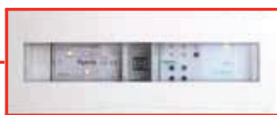
Detail of the porta 4.0 module installed
